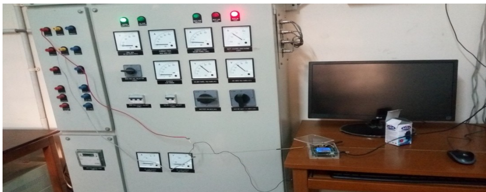
Figure 7.9 Physical implementation of wireless kits to measure voltage
