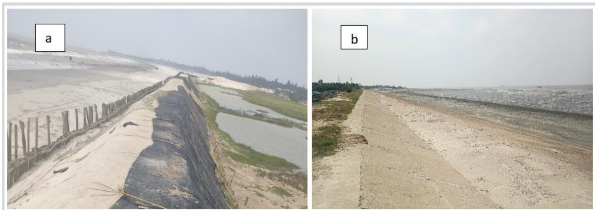
Plate 4.1: (a) Earthen embankment of Sibpur mouza with wood log piling and covered with textile sheets and (b) concrete embankment (Aila Badh) of Beguakhali mouza
