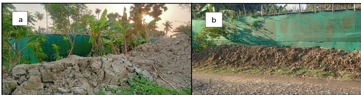
Plate 6.3: Preparation of earthen structures to protect the betel vines from inundation at (a) Bankimnagar and (b) Haradhanpur
