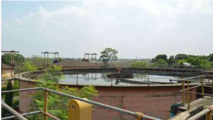
Figure 1.2 Primary settling tank of Barahnagar Kamarhati (KMDA) Waste water treatment plant,
