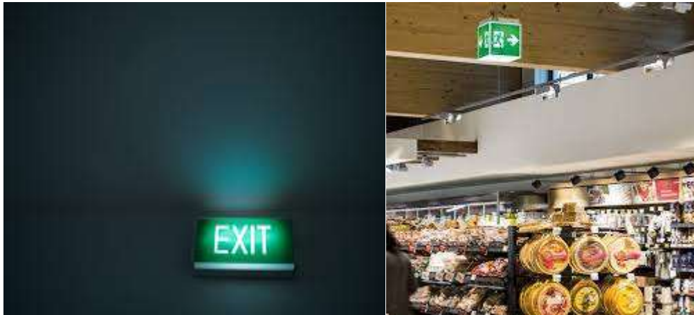
Fig.no 29: emergency exit light in retail space
