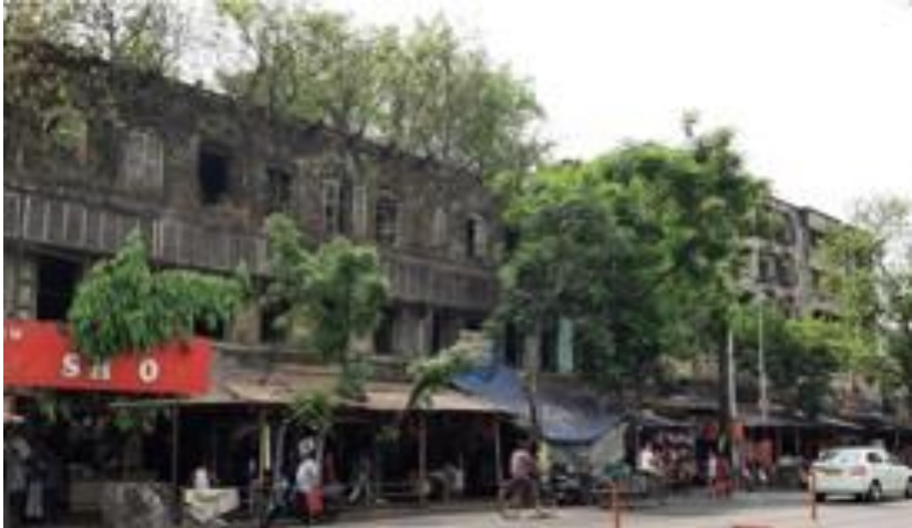
Picture 35: Dilapidated structures, zone I. Source: Author
