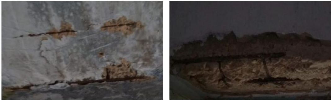
Fig-1.2: Severe Corrosion leads to Spall of Cover Concrete
