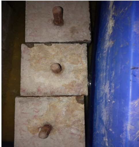
Fig.3.36 Outer surface of Cubes for Half Cell Potentiometer after 4 months acid exposure
