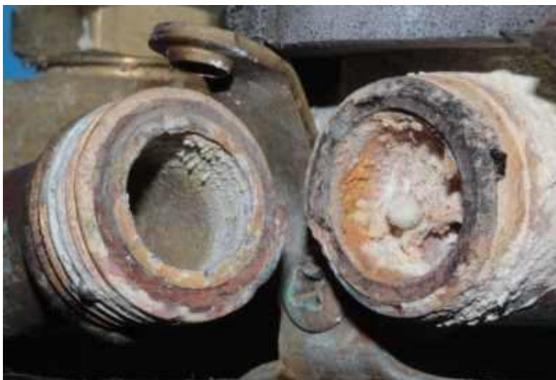
Fig 3: Selective Corrosion of Brass Pipe
