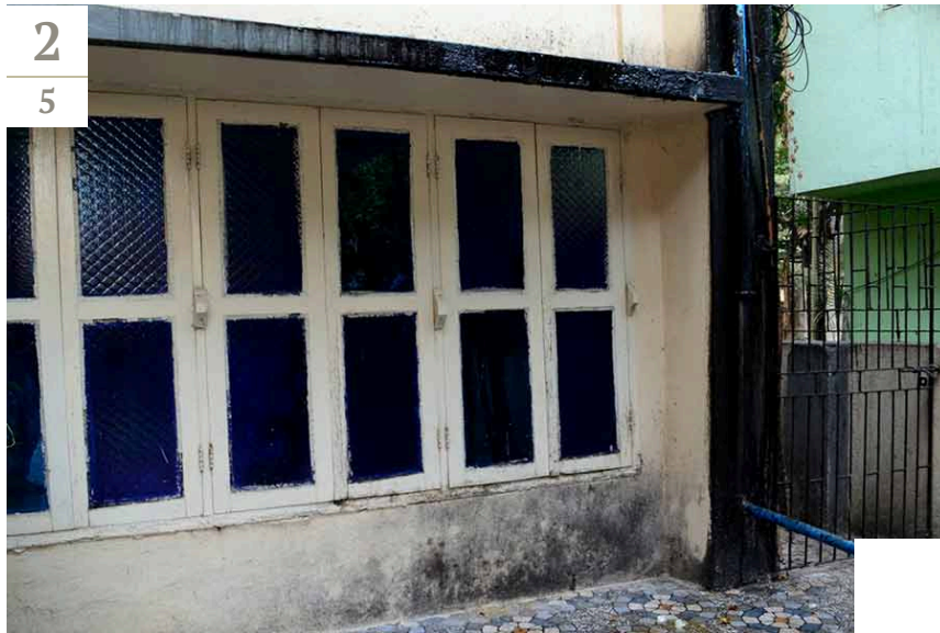
Oil spillage covering the frontal facade of the couple's home in Garia
