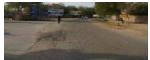
Figure 135 Poor condition of footpath
