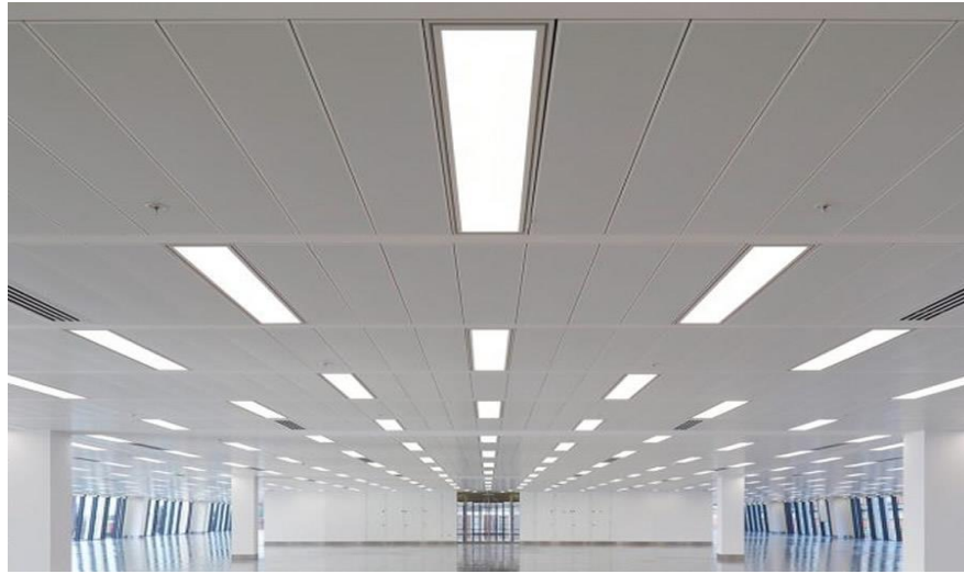
Fig 3.5: Smart LED lighting control system
