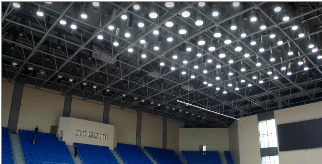
Figure 2.6: Image of Solatube Daylight Pipe installed in an indoor stadium, Beijing
