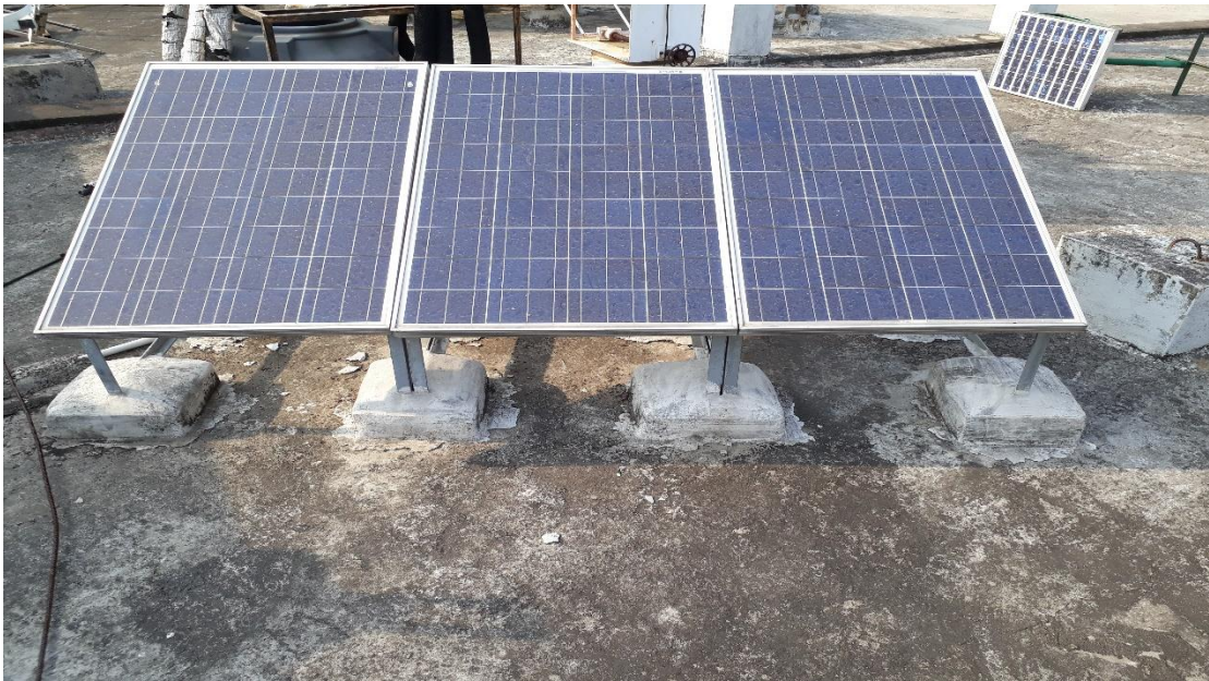
Figure 4.3 Solar Photovoltaic module
