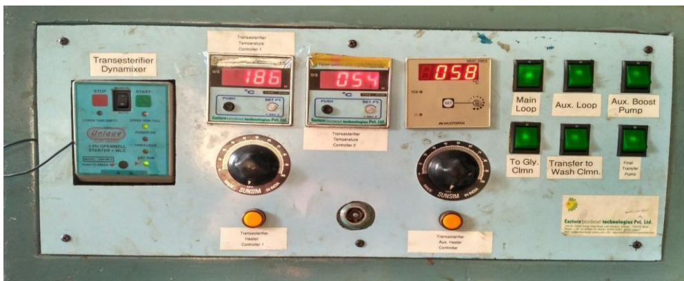
Fig-5.1 : control panel
