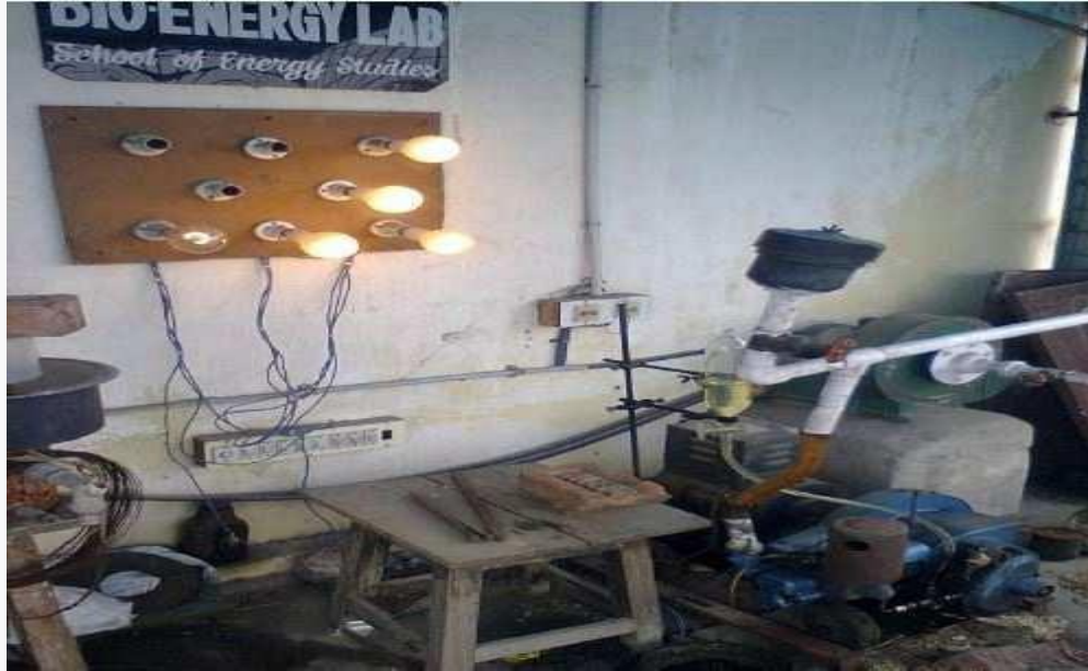
Fig-7.1 :Diesel generator connected with load
