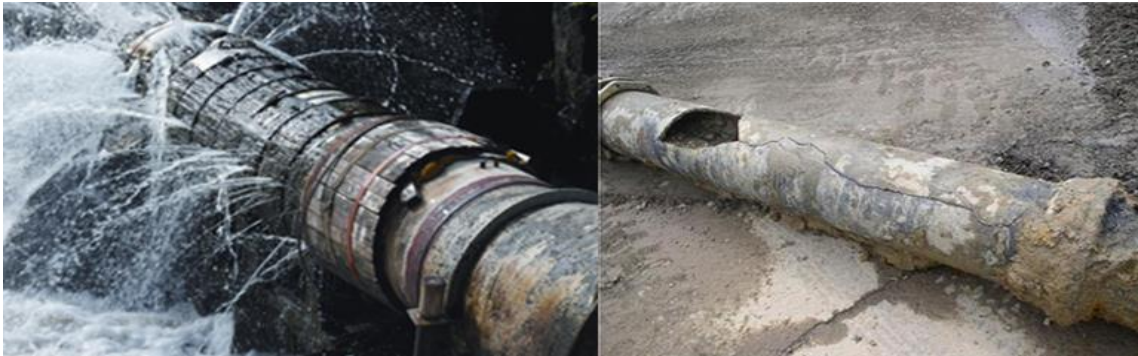
Fig: 2.2. Damaged pipeline due to water hammer phenomena.
