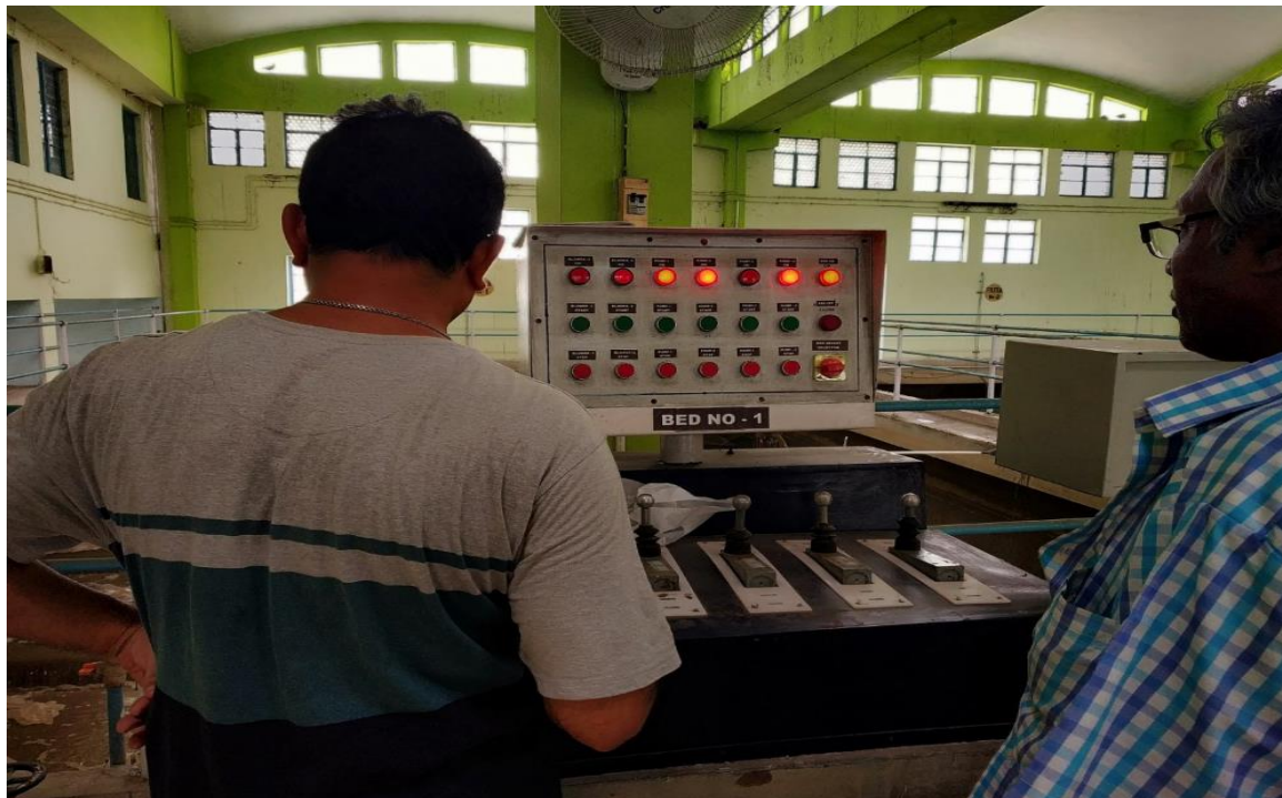
Figure 3.7 Control Panel of Backwashing of Filter Bed
