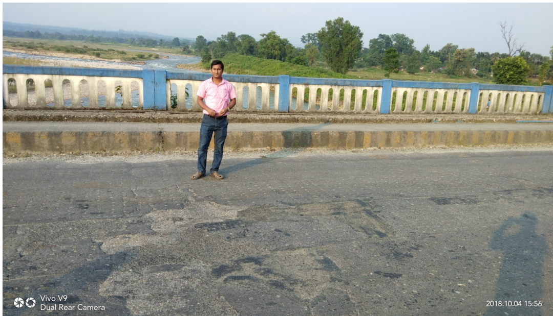
Photograph 4.3: Raveling of road on major bridge portion
