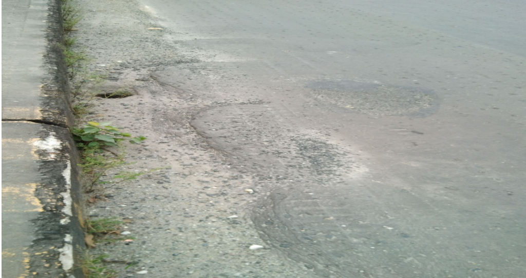
Photograph 4.4: Rutting on project corridor
