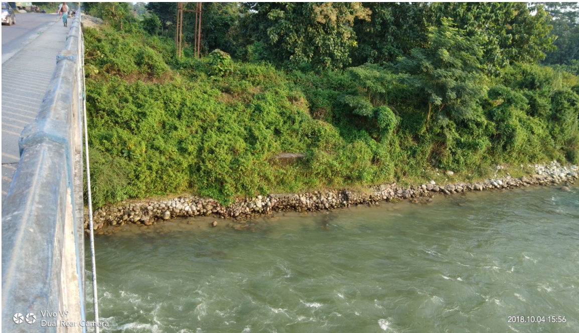
Photograph 4.6: Damage of river protection work
