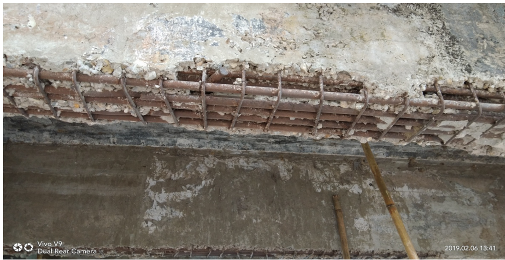
Photograph 4.10: Damage of girder of a minor bridge
