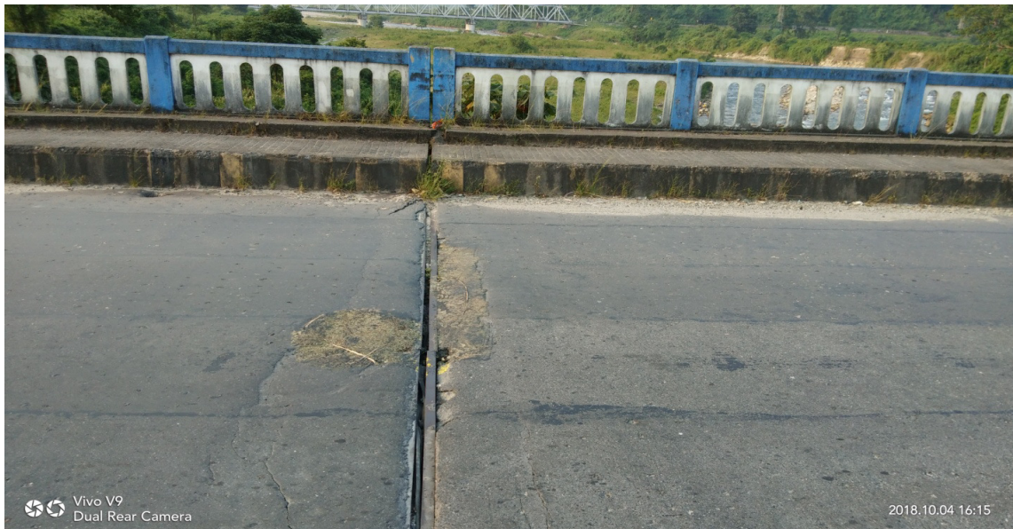
Photograph 4.7: Damage of expansion joint on bridge
