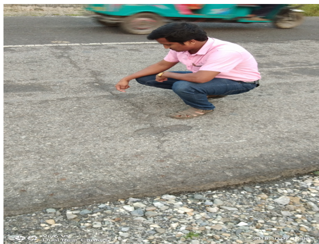
Photograph 4.2: Narrow crack on the project corridor
