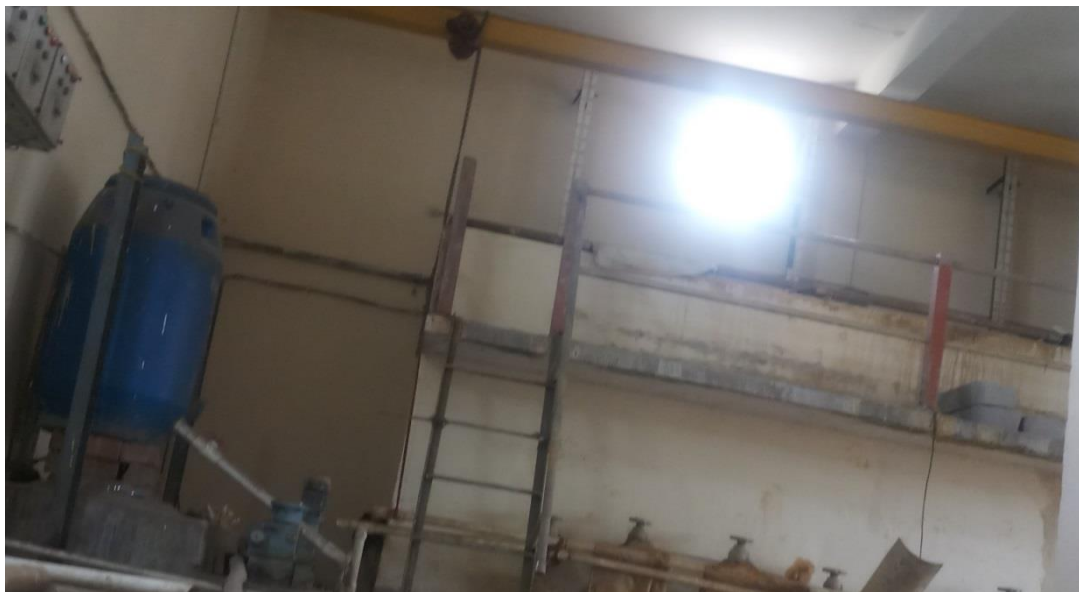
Alum & Chlorination Room
