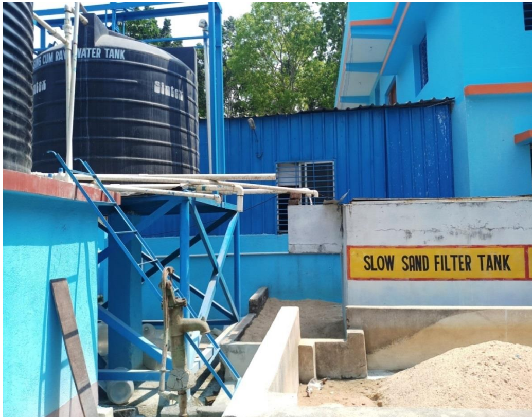
Flocculation Tank & Slow Sand Filter
