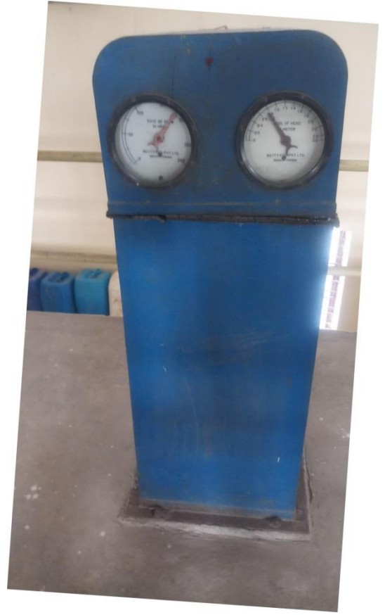
Intake Water Pressure Gauge
