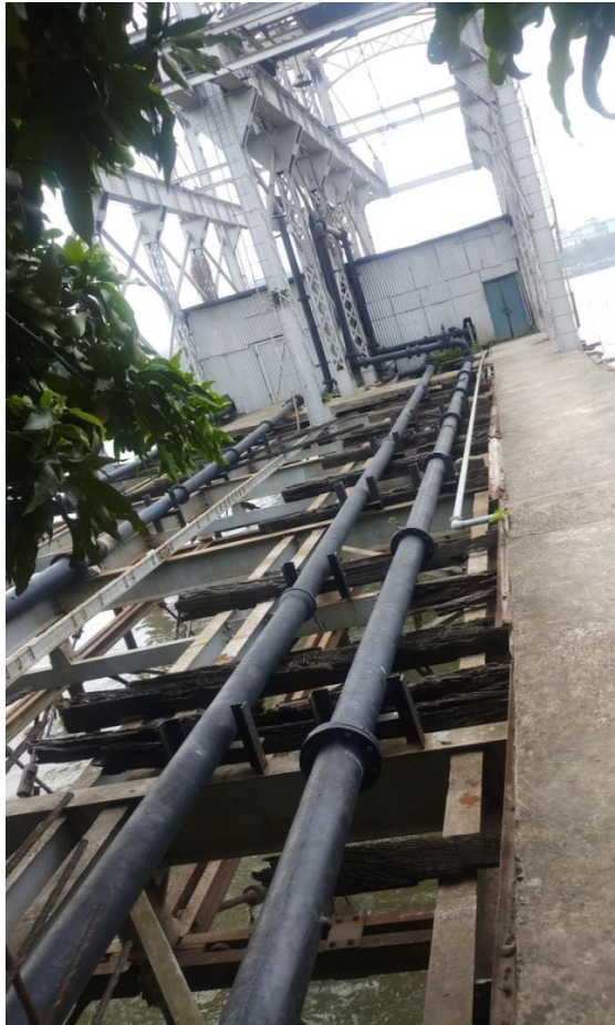
a. Hooghly river intake for Howrah WTP/E.Rly.
