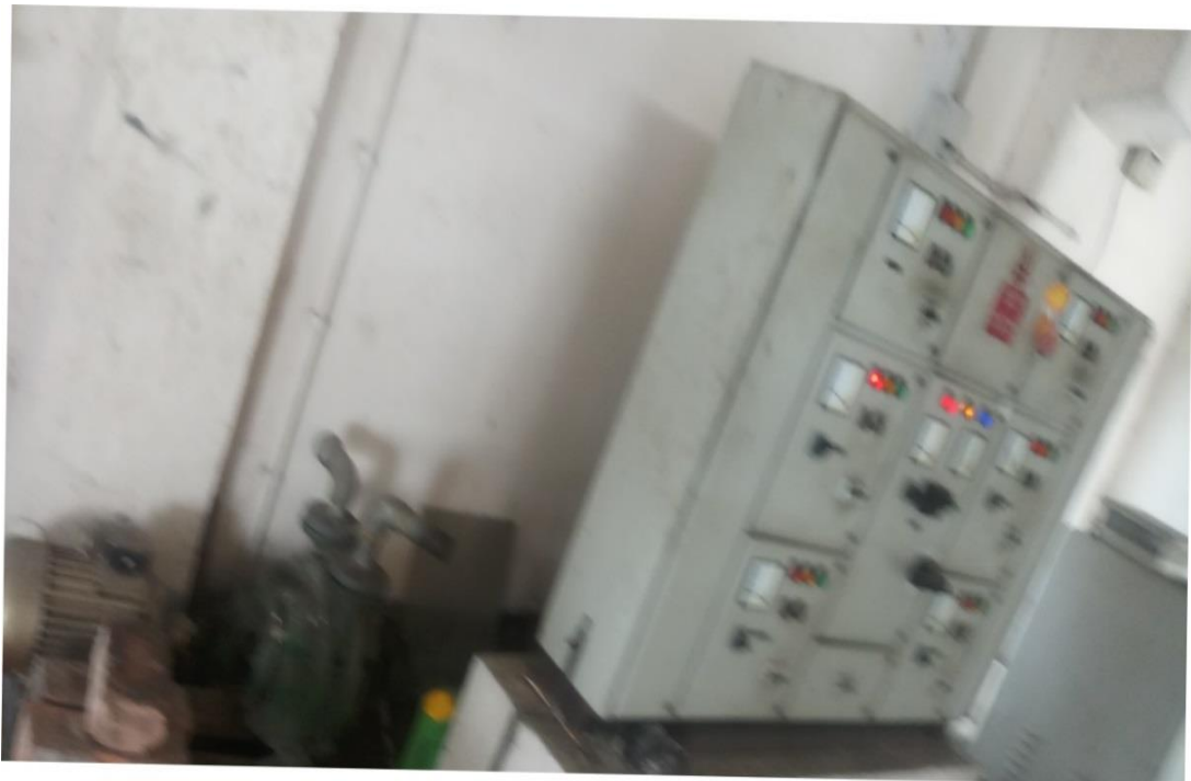
POWER CONTROL ROOM
