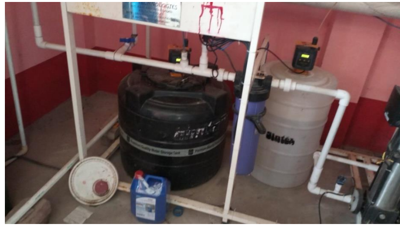
RO Unit of north 24 Parganas (Hingaljan)
