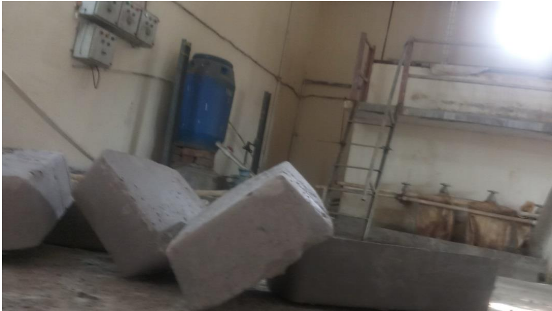
Alum & Chlorination Room
