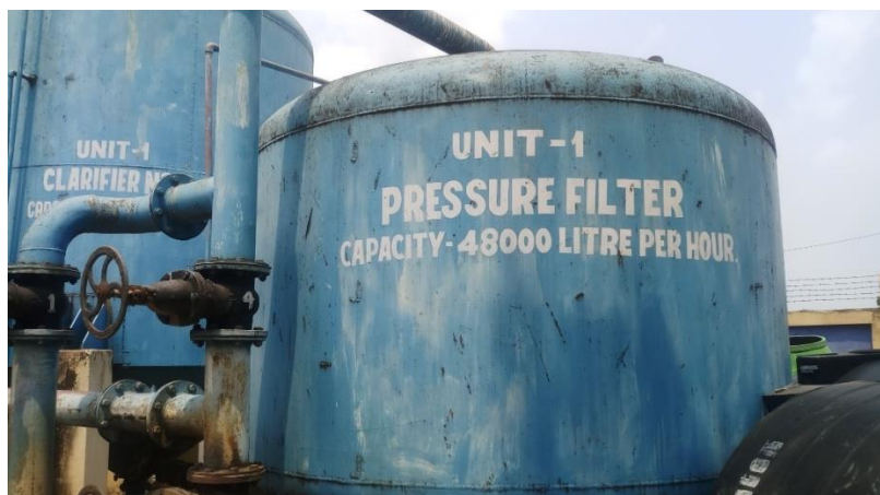
Pressure filter(HWH-WTP) Figure-5.5.5
