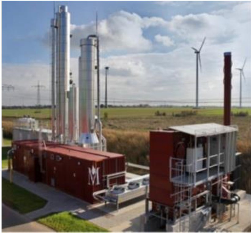
Conventional Water Scrubbing for biogas purification
