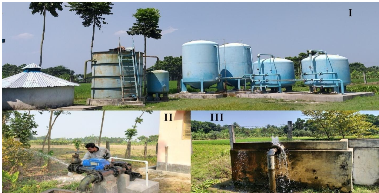
Fig 8.3: (i) Kola Plant (ii) Sample collection (iii) Overflow of sludge tank
