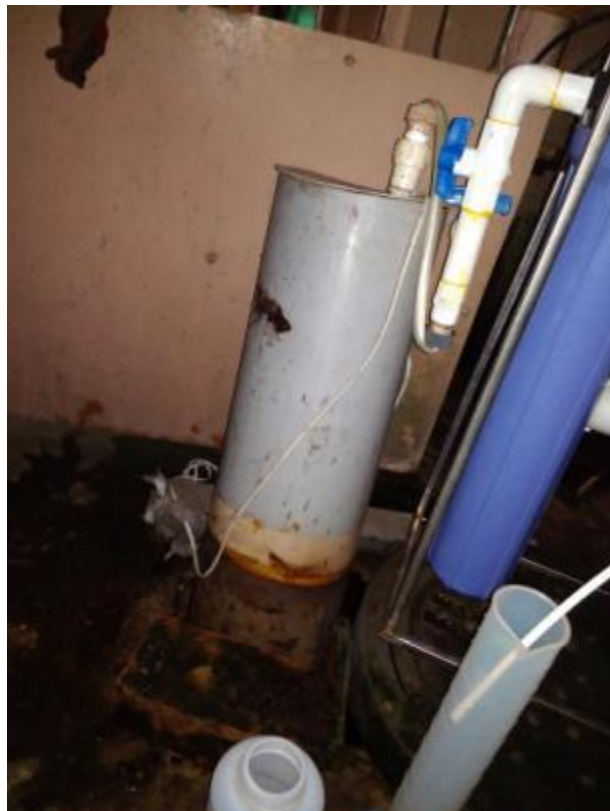
Fig. 16: Flexible Pipe connecting perforated pipe and PLE machine is subjected to tension due to upward movement the perforated pipe
