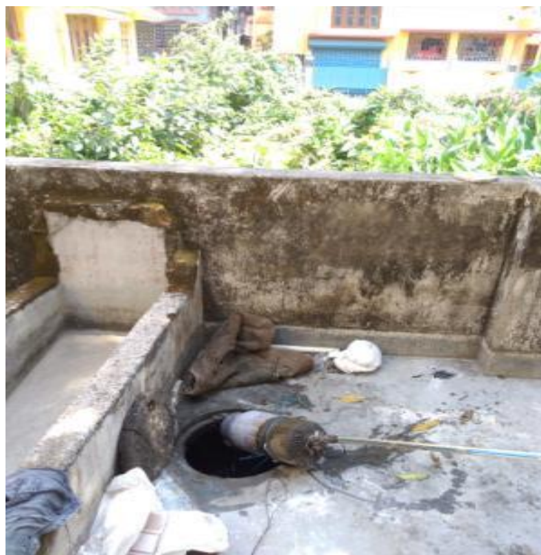
Fig. 71: Perforated pipe after three days of operation
