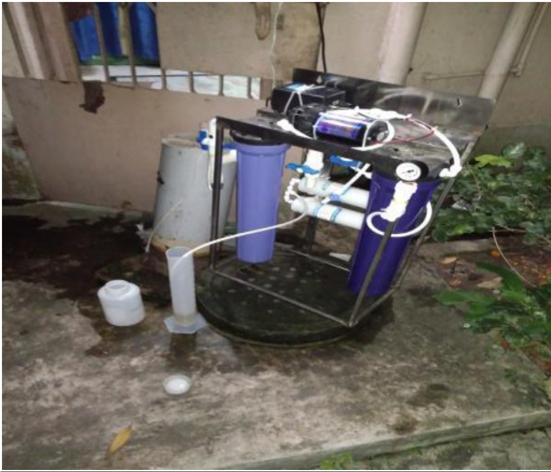
Fig. 17: Installation at Site 1. for 2 nd Cycle
