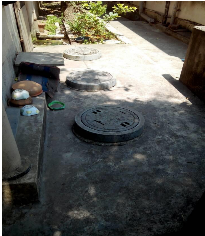
Fig. 2: Septic Tank at Site 1.
