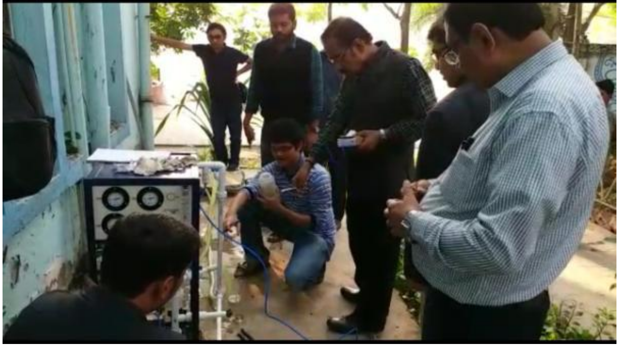
Fig. 33: Installation at Site 2. For 2 nd Cycle
