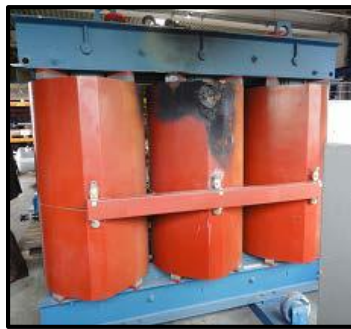
Fig. 3.2. Partial Discharge on Dry-type Transformer.
