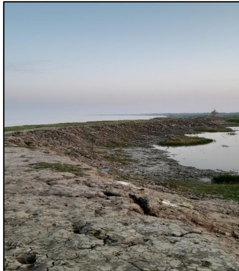
Photograph. 3: Breached embankment in Boatkhali-Dhablat, Sagar Island
