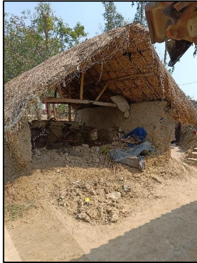
Photograph.7: A dilapidated house in Ghoramara after Cyclone Yaas in 2021
