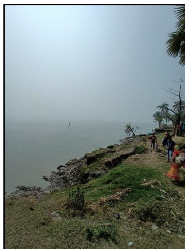
Photograph.6: State of embankment in Ghoramara island
