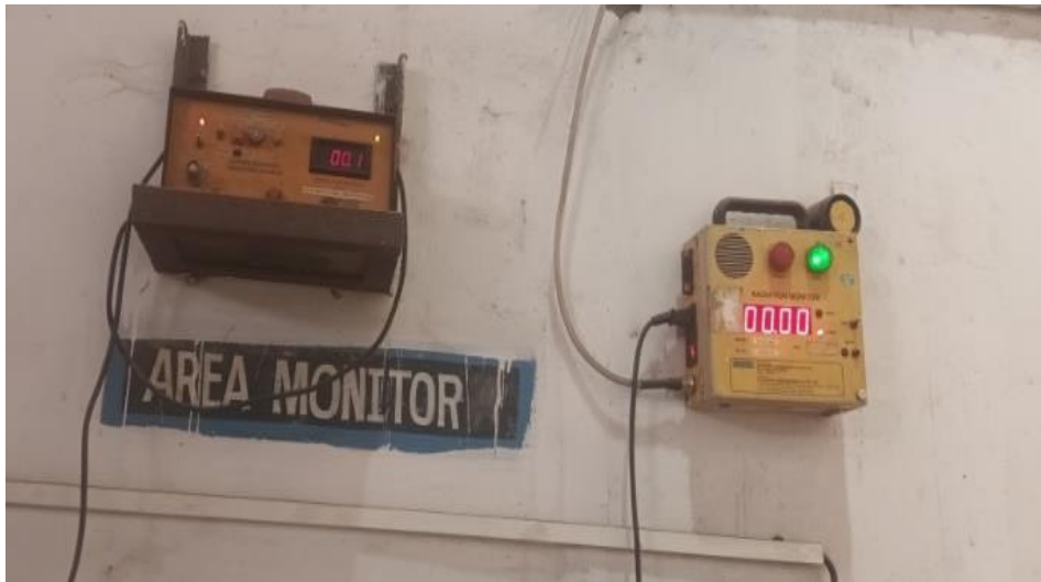
Fig. 4.2: Area Radiation Monitor
