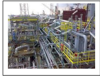
Figure 9-15: Shell and Piping
