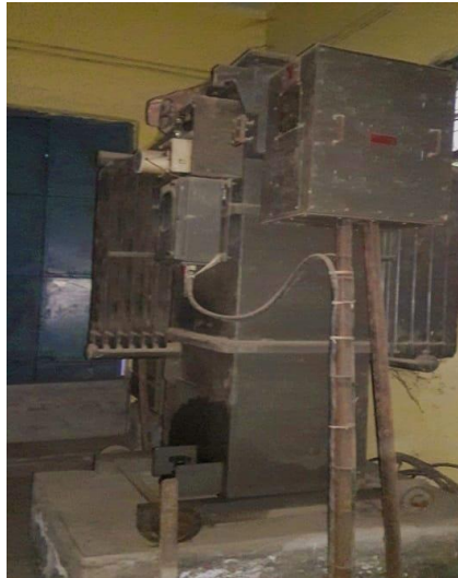
Fig. 2.5 (a) High Voltage on-load Voltage Regulator (VR).
