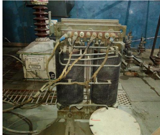
Fig. 2.5 (b) High Voltage Auto-transformer.
