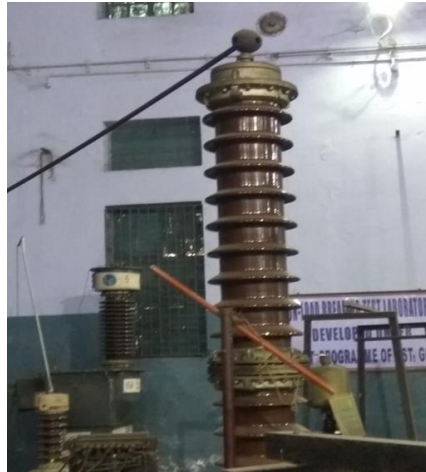
Fig. 2.6 High Voltage Potential Divider.
