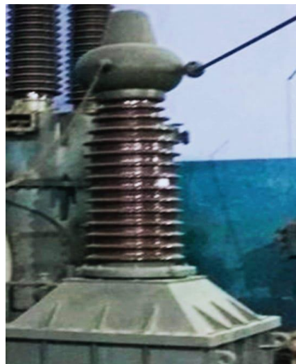
Fig. 2.5 (c) High Voltage Testing Transformer.
