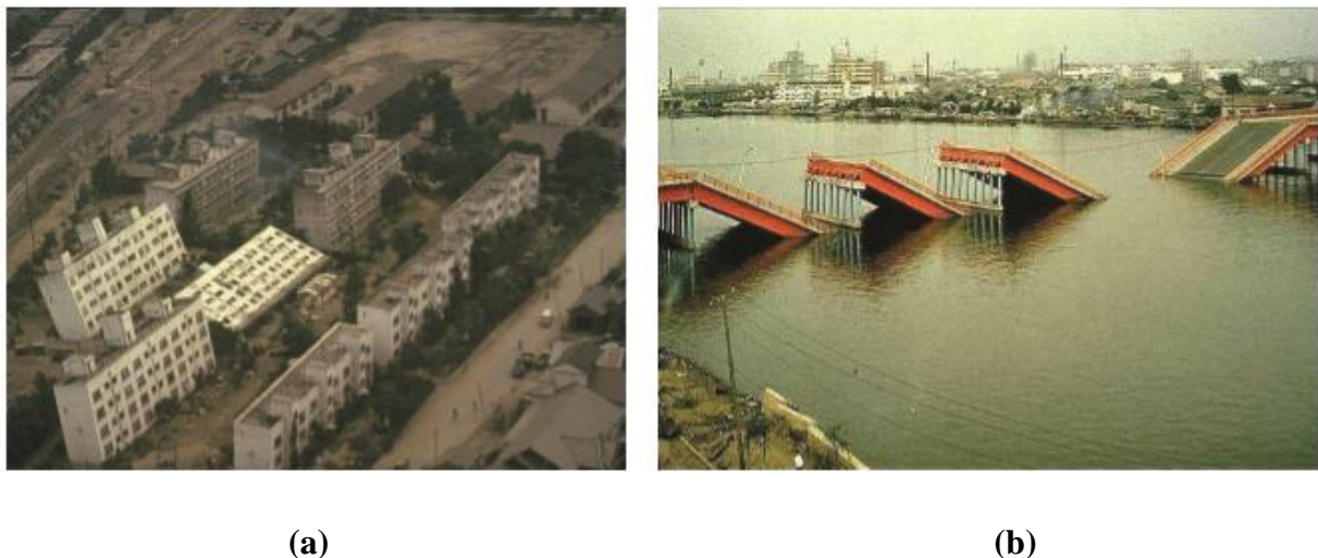
Fig. 1.4 Failures of a Kawagishi-cho apartment and b Showa bridge following the 1964 Niigata Earthquake due to liquefaction (Choudhury et al. 2014)
