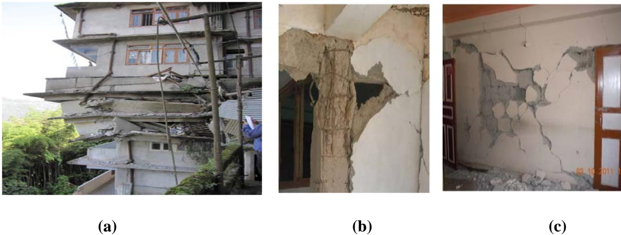
Fig. 1.11 a Structural failure of two intermediate storeys of 9-storied building b failure pattern of column and c failure of infirm masonry wall at Gangtok during 2011 Sikkim earthquake (Rai et al. 2012)
