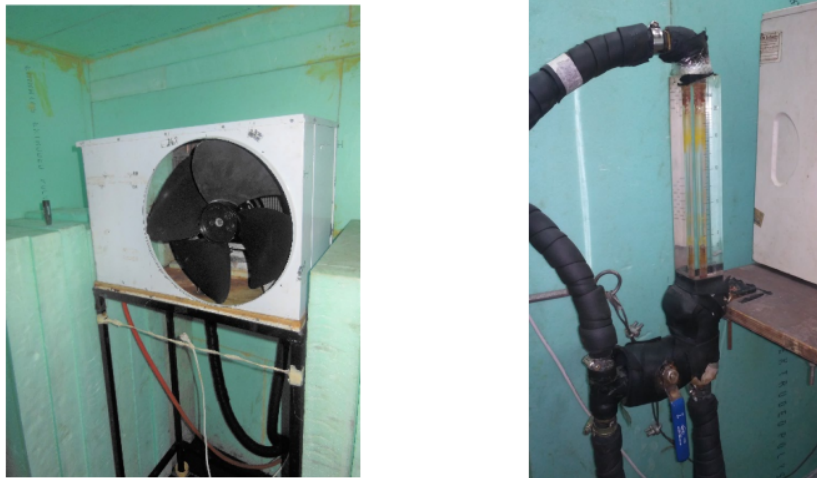
Fig. 2.13 Heat Exchanger Fan Coil unit along with rotameter-based flow control
