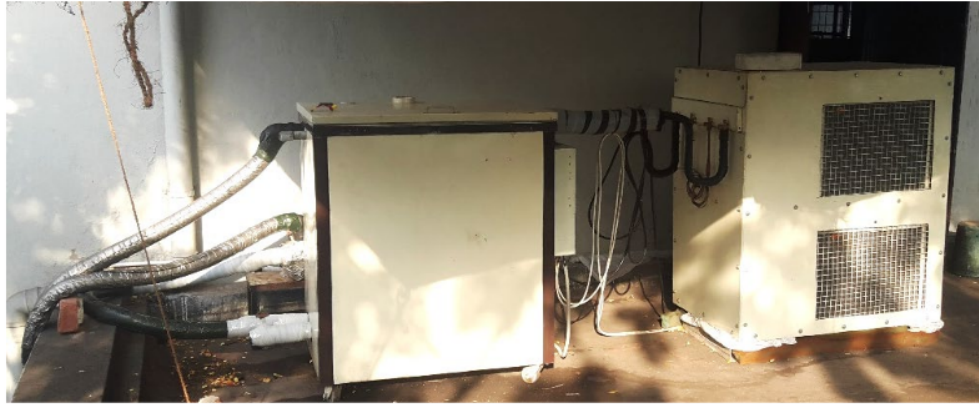
Fig. 2.14 Sub-zero dilute calcium chloride solution based chilled storage unit
