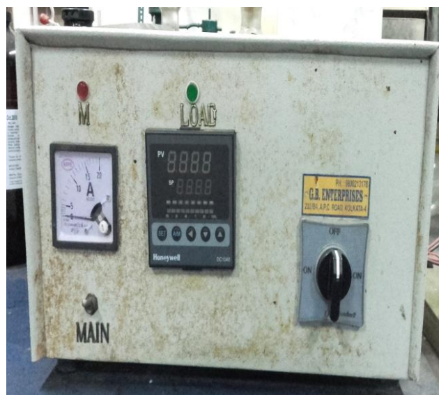
Fig 4.3: PID Temperature Controller
