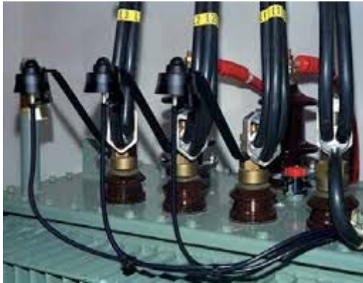
Metal oxide LV surge arrester
