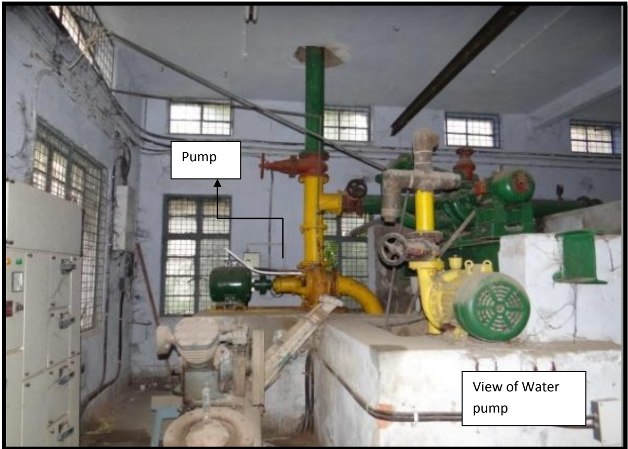
Fig 3.1.5, A view of pump system in ground floor
