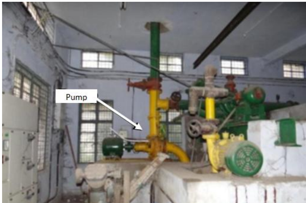
Fig. 4.7: Water Pump for the flow through channel
