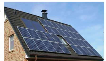
Solar Panels on sloping roof
