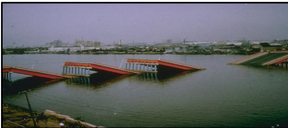
Fig 1.8 : Failure of Showa bridge following the 1964 Niigata earthquake
