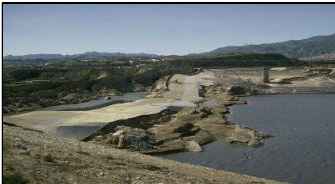
Fig 1.6 : Liquefaction failure of upstream slope of lower San Fernando Dam in 1971 San Fernando earthquake
