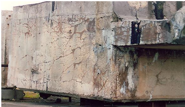
Figure – 2.46: Bacterial attack on concrete.
