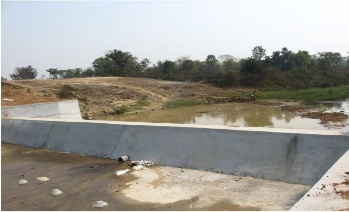
Photo 10.1 : Initial river water condition just after construction of Check Dam in summer, 2014.
