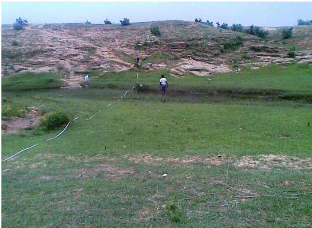
Photo 9.1: The length measurement for check dam layout of prior begin the construction work
