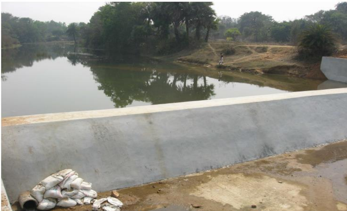
Photo 10.2 : Increase in river water condition just after week of construction of Check Dam in summer, 2014.
