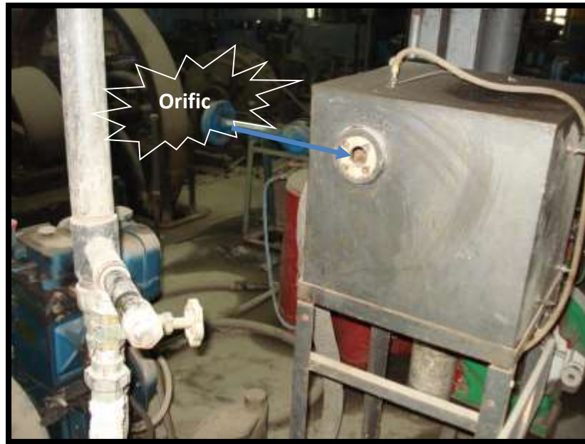
Plate 5.4: Surge tank fitted with orifice
