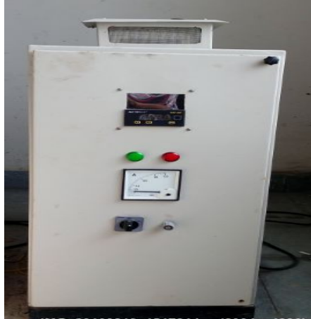
Fig 4.2.11: Control panel for the shake table for rpm control
