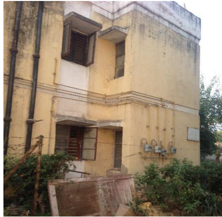
Plate 5.6 CNG connection in the CPWD colony Source: Field Survey
