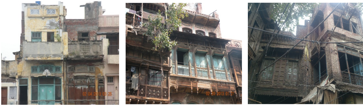
Plate 4.3: Poor Condition of Buildings, Katra Dullo, Amritsar
