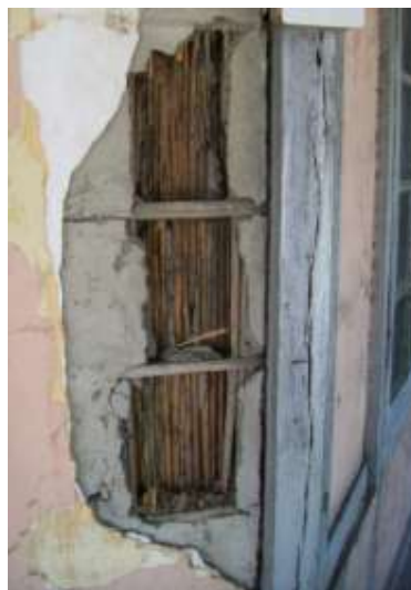
Figure 2.9: Wattle and Daub Technique Used in the Walls of a Traditional Assam-Type House (Source: Author)
