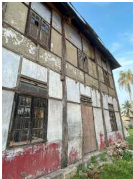
Figure 2.5: Side View of an Assam-Type House Illustrating the Core Principle of Assam-Type Construction: Strong Base, Flexible Midsection, and Lightweight Top (Source: Author)
