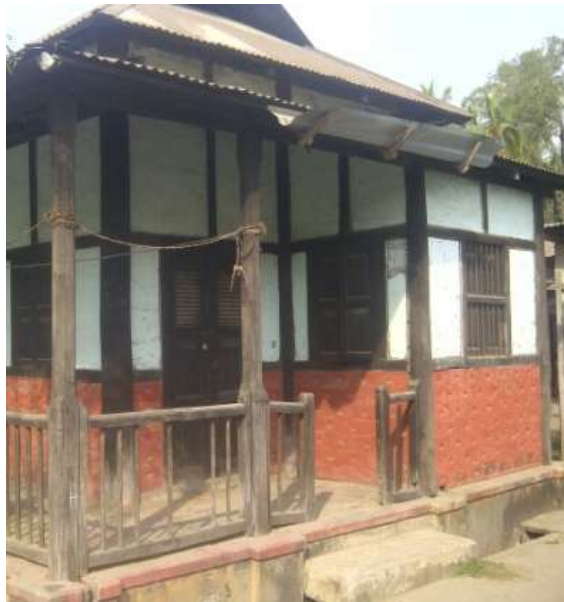
Figure 2.10: Lower Brick Wall and Upper Wood-Bamboo-Ikra Section Using Wattle and Daub in an Assam-Type House (Source: Shermin 2017)
