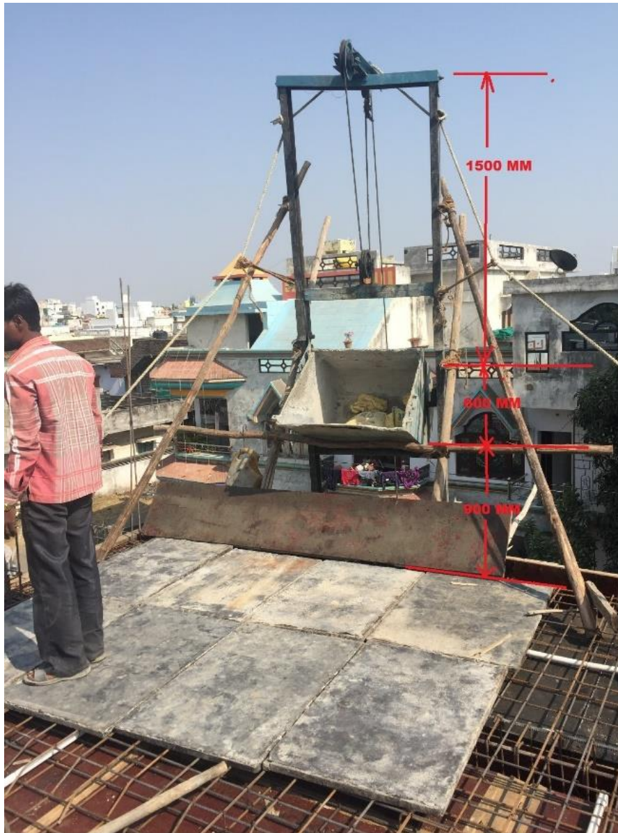
Figure (i) Real time elevator with vertical distance (at first floor)
