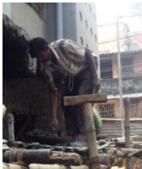
(e) Picking mortar for plastering (to apply on wall) (for outside plastering) (PL-5)
