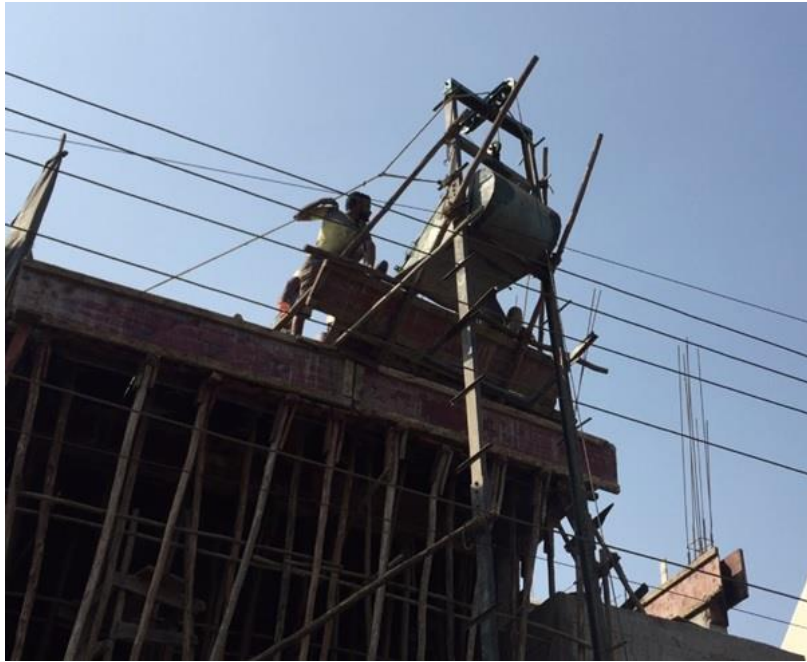
Figure (ii) Real time Elevator (view from ground)
