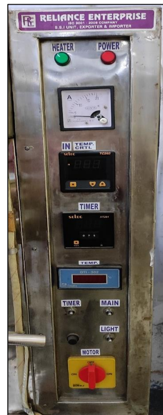
Fig 3: FBD control panel
