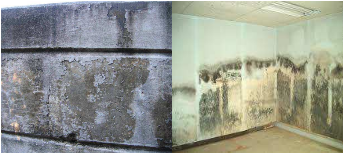
Fig. 1.1 Surface of concrete walls covered and affected by fungal biofilm (Kurth et al., 2008).
