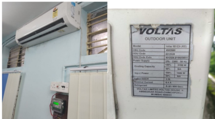
Figure 5.2: Photograph of Voltas Make 1.5 Ton capacity AC systems with its specification
