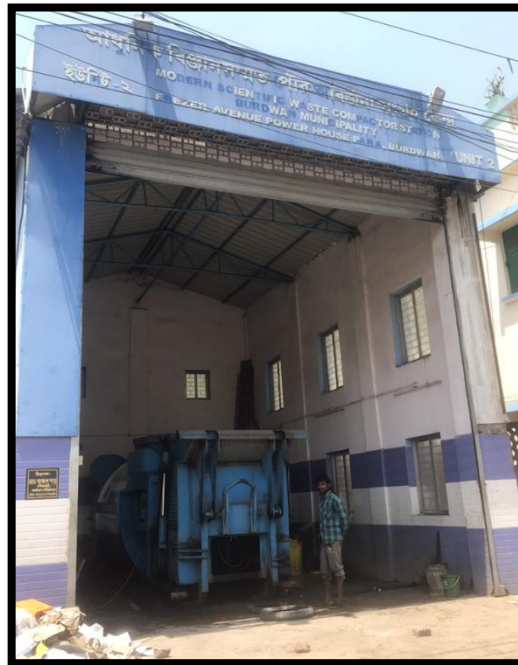
Photo.5.2.1. The Solid Waste Compactor Station (Unit-2)
