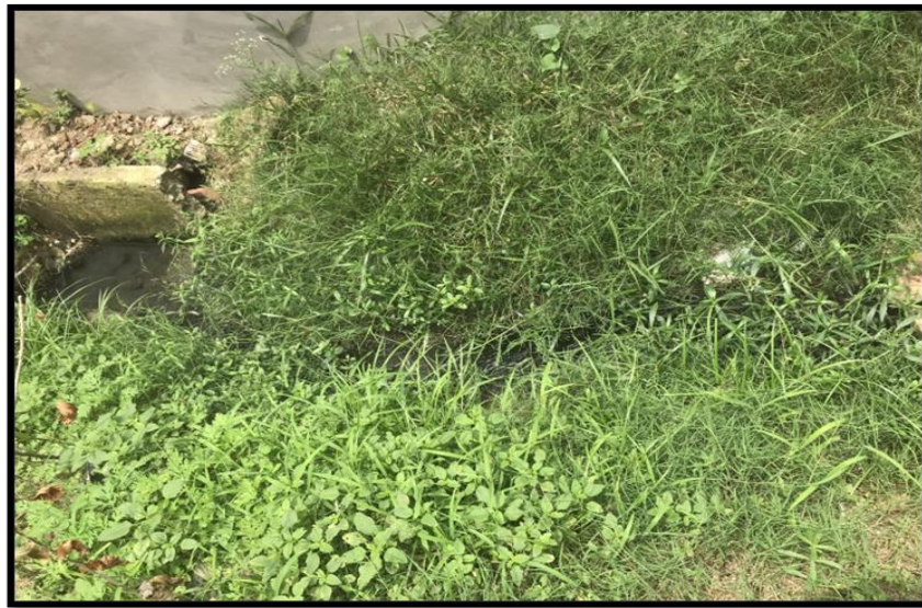
Photo: 5.3.7. Drain adjacent to Ananda Pally Road (Pond) Ward No.10
