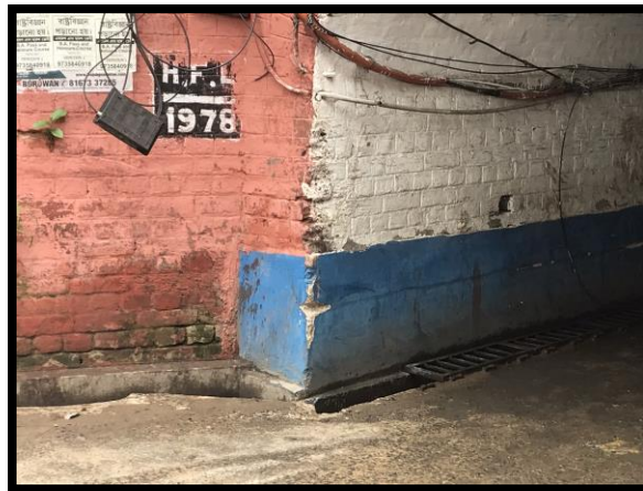
Photo.5.3.36. The Highest Flood Level Marked at the Kalna Gate Sub-Way (Source: Field Survey,2023)
