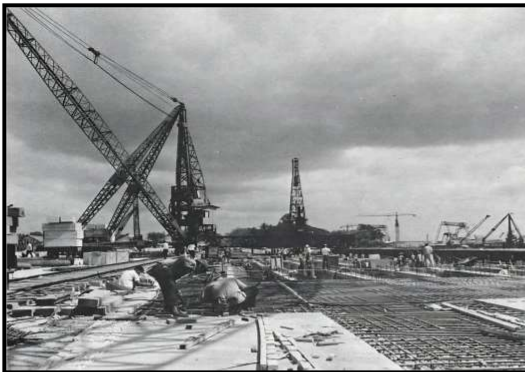
Construction of Container Facilities at Singapore Port with the assistance of the World Bank
